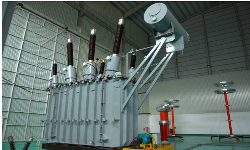
Transformer under testing
