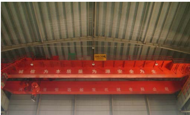
200T Traveling Crane
